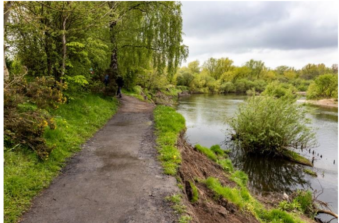
Riverbank erosion at Baron's Haugh © David Palmar
